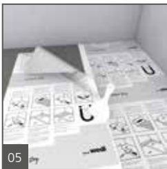
05 Spread flat all wedi Sealant 620 using a putty knife. Cross joints should be avoided.
